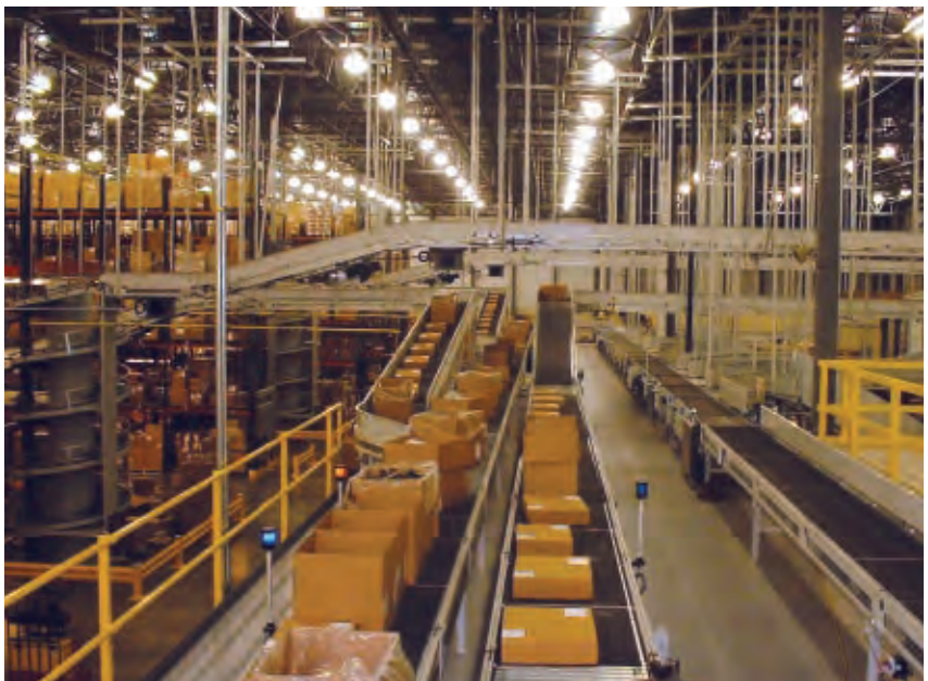
Automated materials handling technology and new processes are enabling multi-channel retail distribution from one facility.
